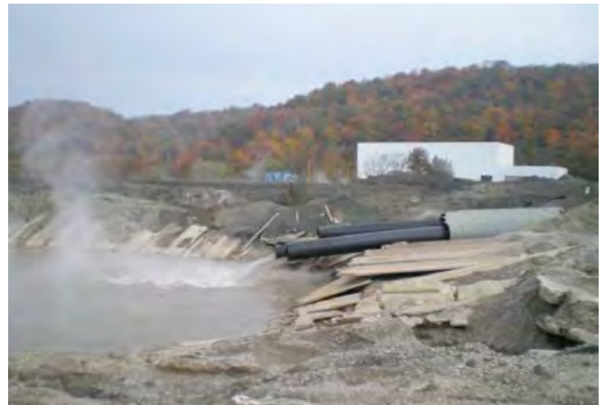
Sluice lines entering “Pond 5” at the J.M. Stuart Station, located in an Ohio River flood zone. Pond 5 was found by an EPA assessment to be in “poor” condition, and to pose a “significant” hazard to the surrounding area. Image: U.S. Environmental Protection Agency
