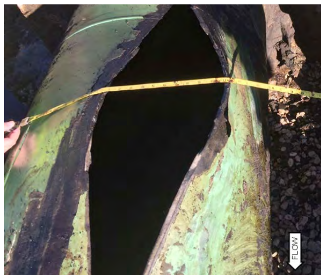
This rupture in the Keystone Pipeline near Amherst, South Dakota, led to the spill of approximately 5,000 barrels of oil. 113 Image: National Transportation Safety Board
